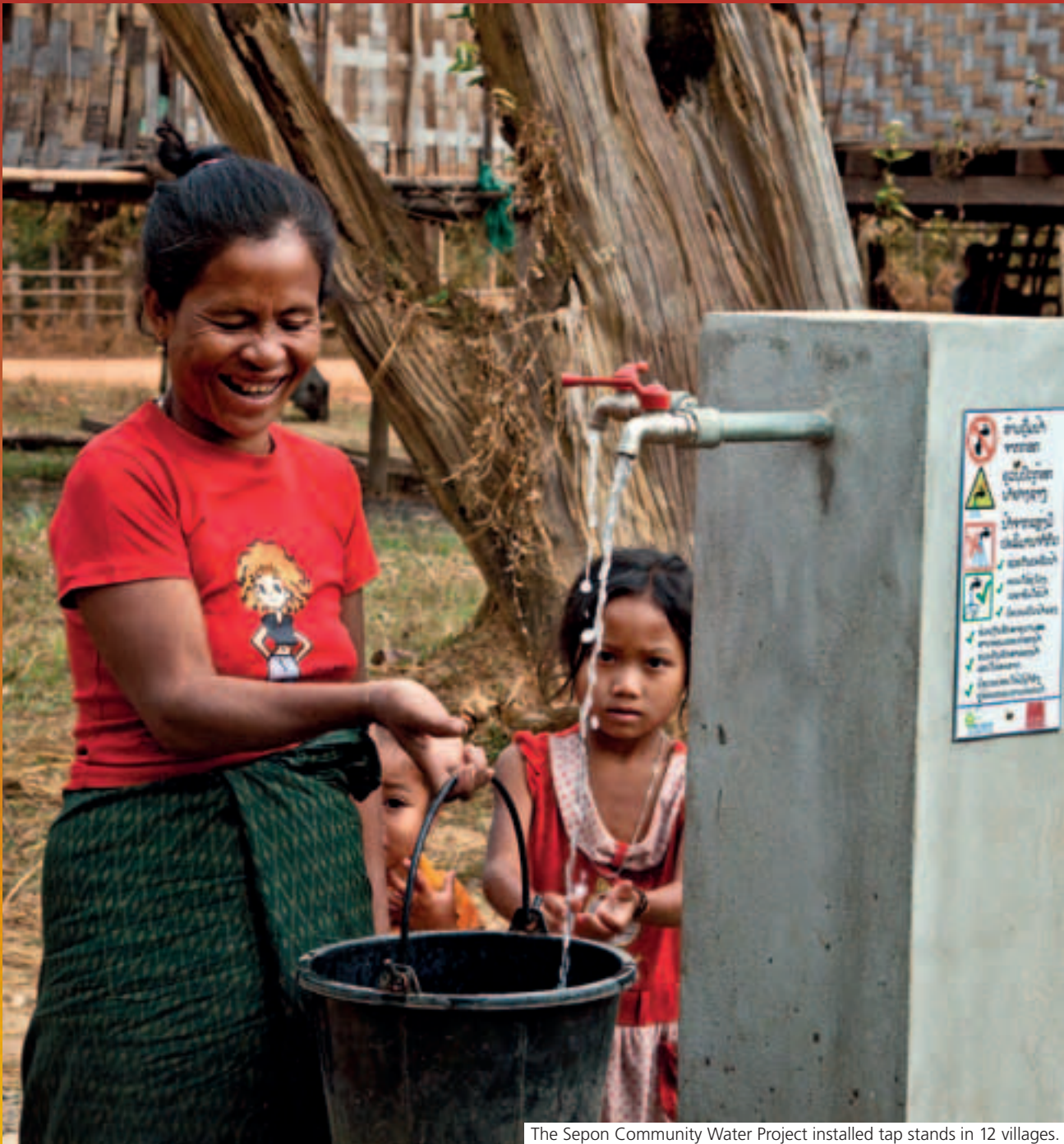
The Sepon Community Water Project installed tap stands in 12 villages.
