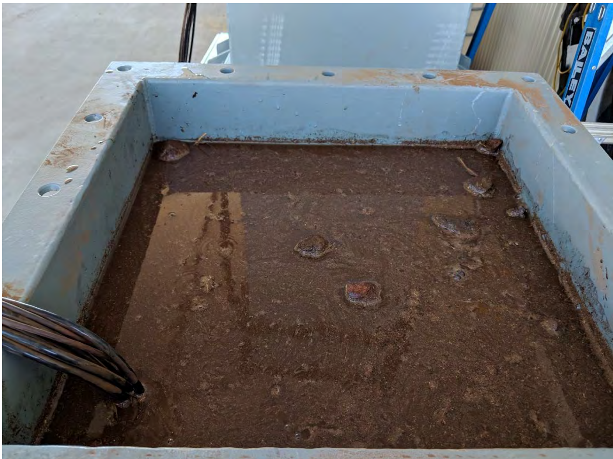
Photograph 2 Ponding of water on the trials
