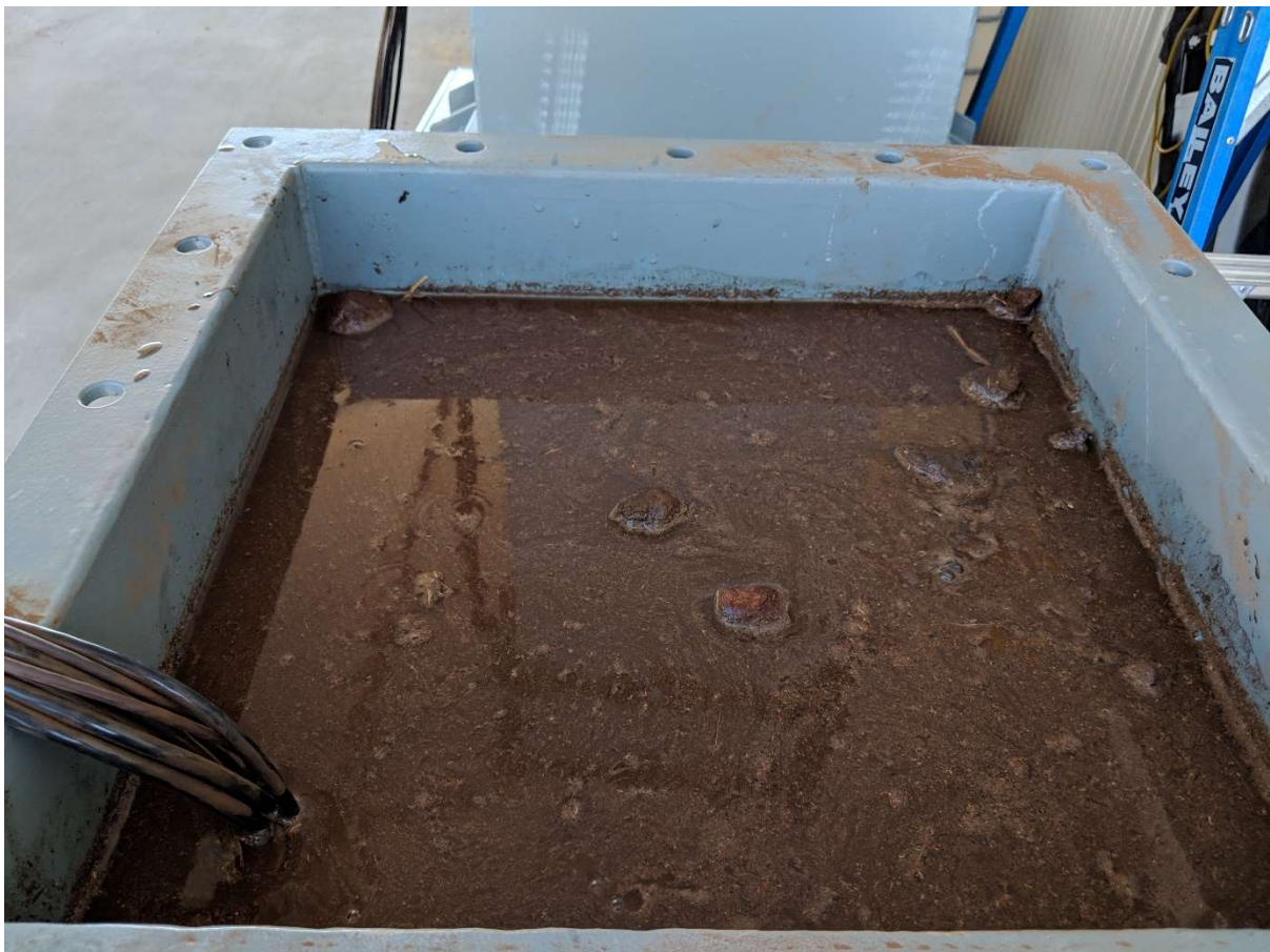
Photograph 2 Ponding of water on the trials
