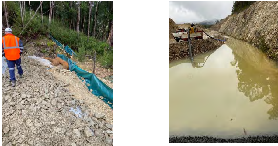
Figure 2-2. Implementation of improved sediment retention infrastructure following discharge of turbid water to the Stitt River (left), and use of pumps to transfer turbid water to the TSF (right).
