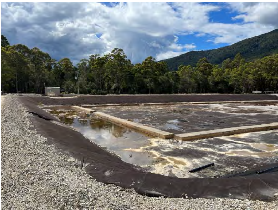
Photograph 18 – seepage return pipeline previously located on SCP liner has caused damage to the lining system and will require repair.
