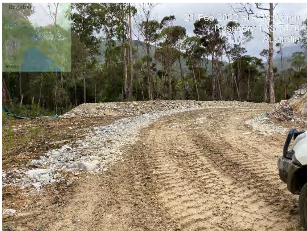
Photograph 33 – bund formed across the outlet to the diversion channel (to be removed once stage 2 works are complete).
