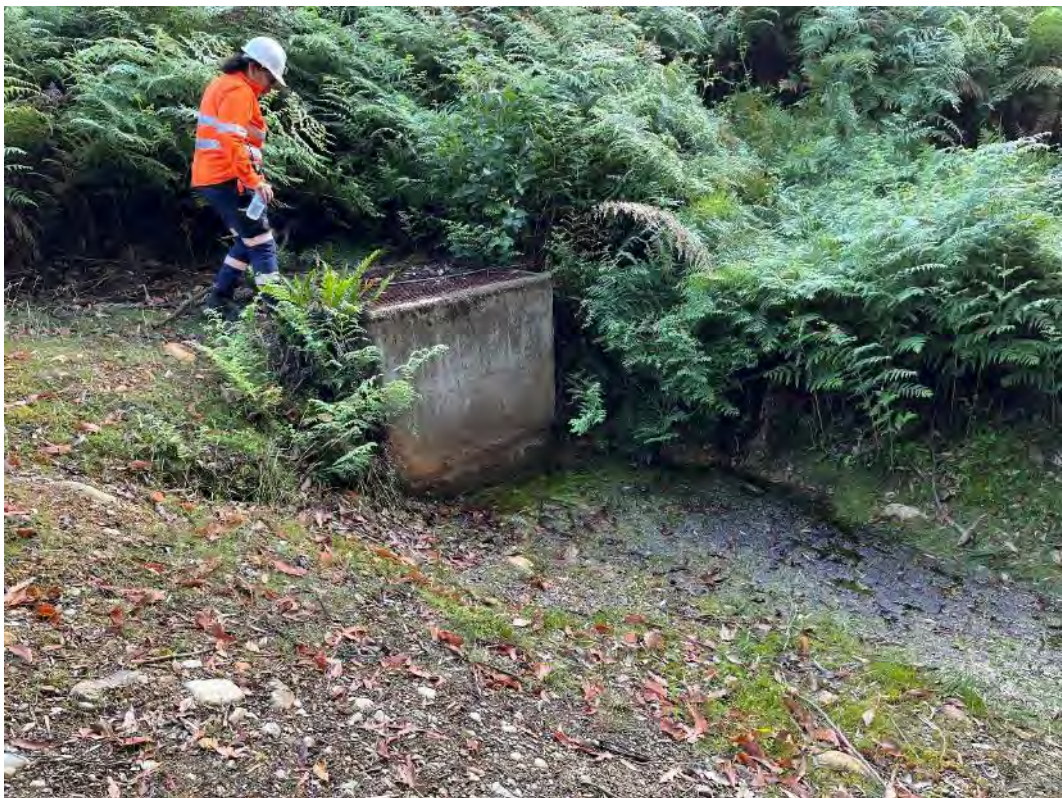
Photograph 38 – Leaking pit downstream of the railway line near BDSP 01.
