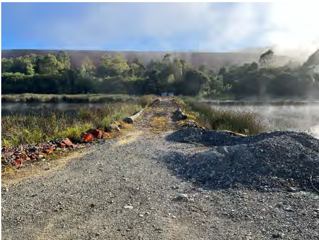
Photograph 44 – Polishing Pond – overgrown cell 3/4 dividing embankment slashed. Vegetation at internal spillway (background) should also be removed.
