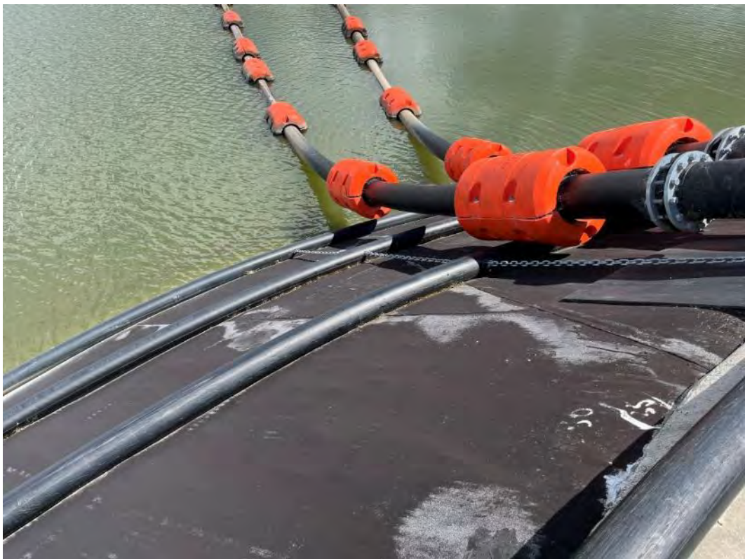
Photograph 8 – damage to Stage 1 liner on upstream face of eastern embankment due to dragging of pipeline.
