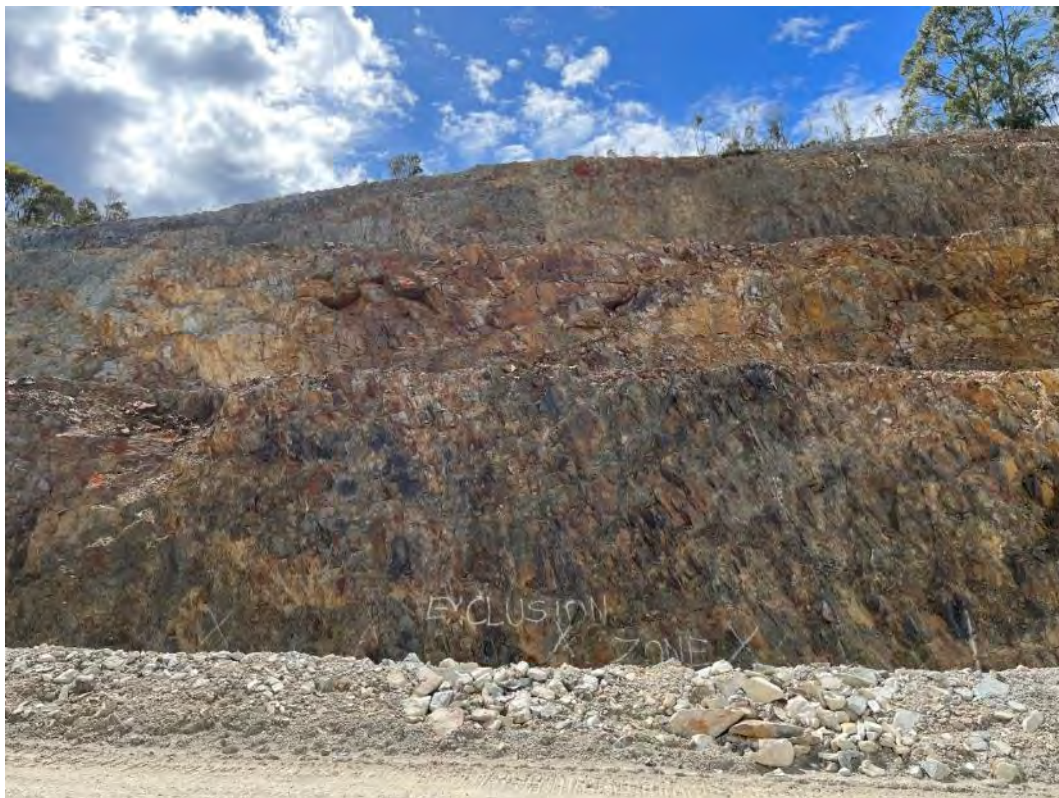
Photograph 32 – loose rock in western cut face of the diversion channel
