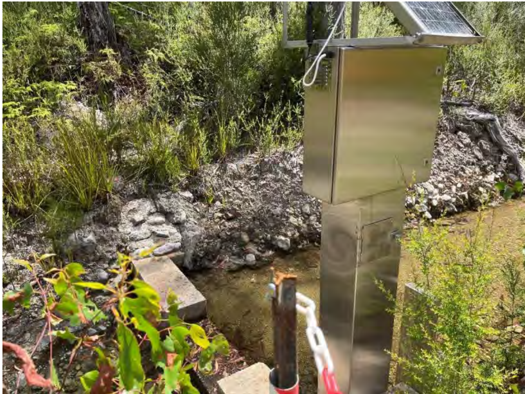
Photograph 1 – Flow measuring weir installed at eastern end of CWDD
