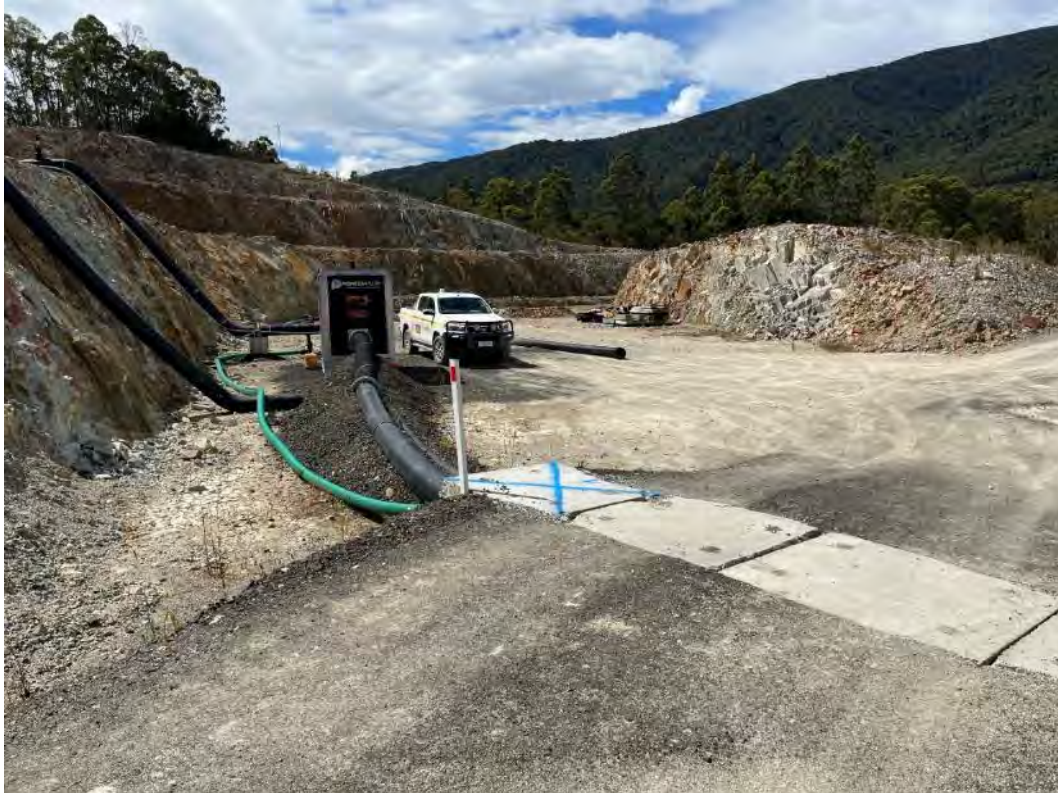
Photograph 27 – spillway, pump for sprinkler system will need to be removed as part of Stage 2 works
