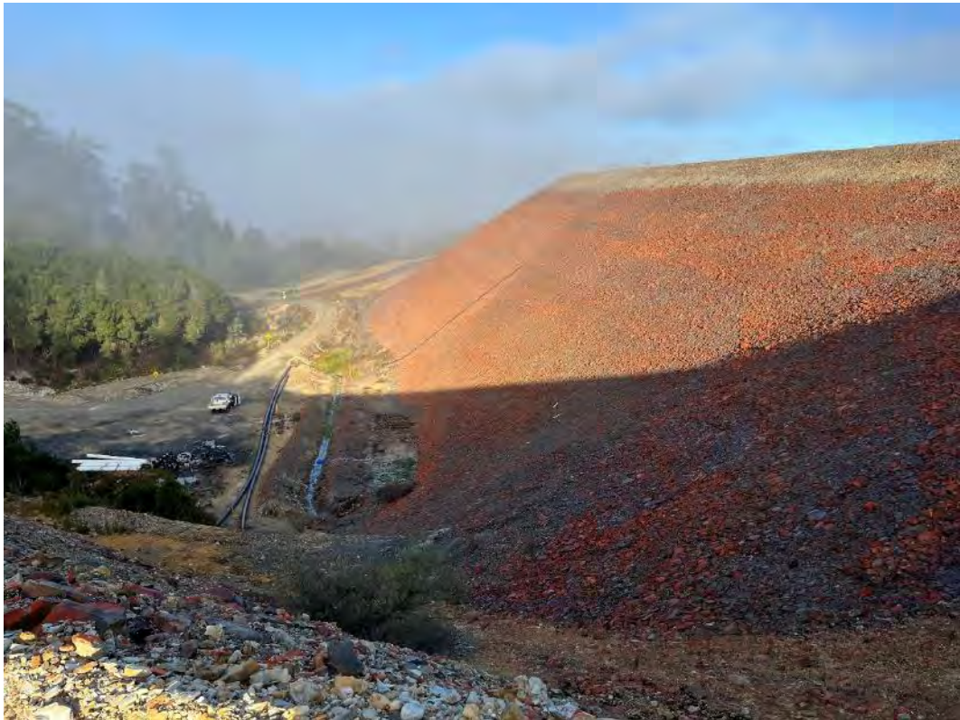
Photograph 3 – Downstream slope western buttress and dense vegetation in toe drain, looking north.
