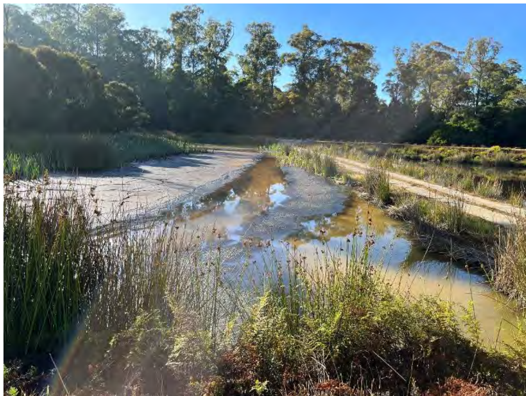
Photograph 39 – Polishing Pond Cell 1. Large amounts of sludge have accumulated within several cells.
