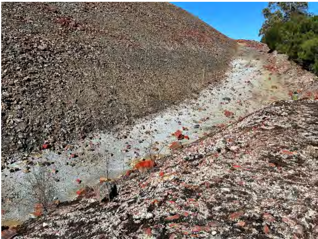
Photograph 10 – Downstream slope of northern embankment, looking west towards Levee Embankment, note salt precipitation.
