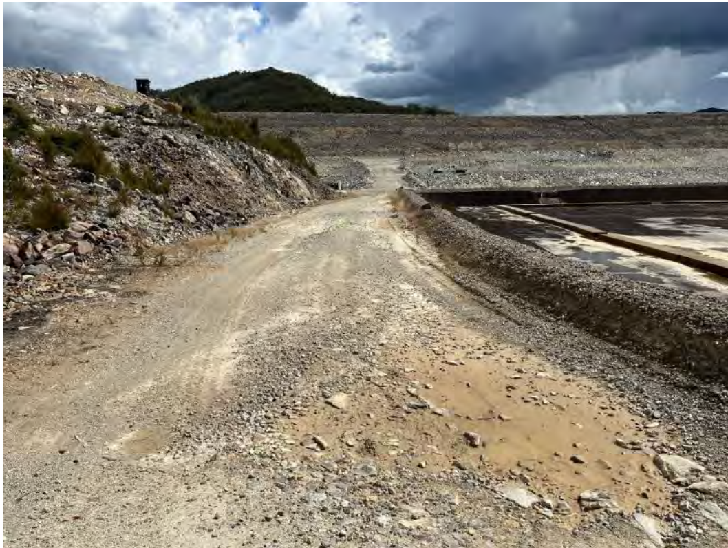
Photograph 17 - Low points on eastern crest of the SCP. Maintenance required.
