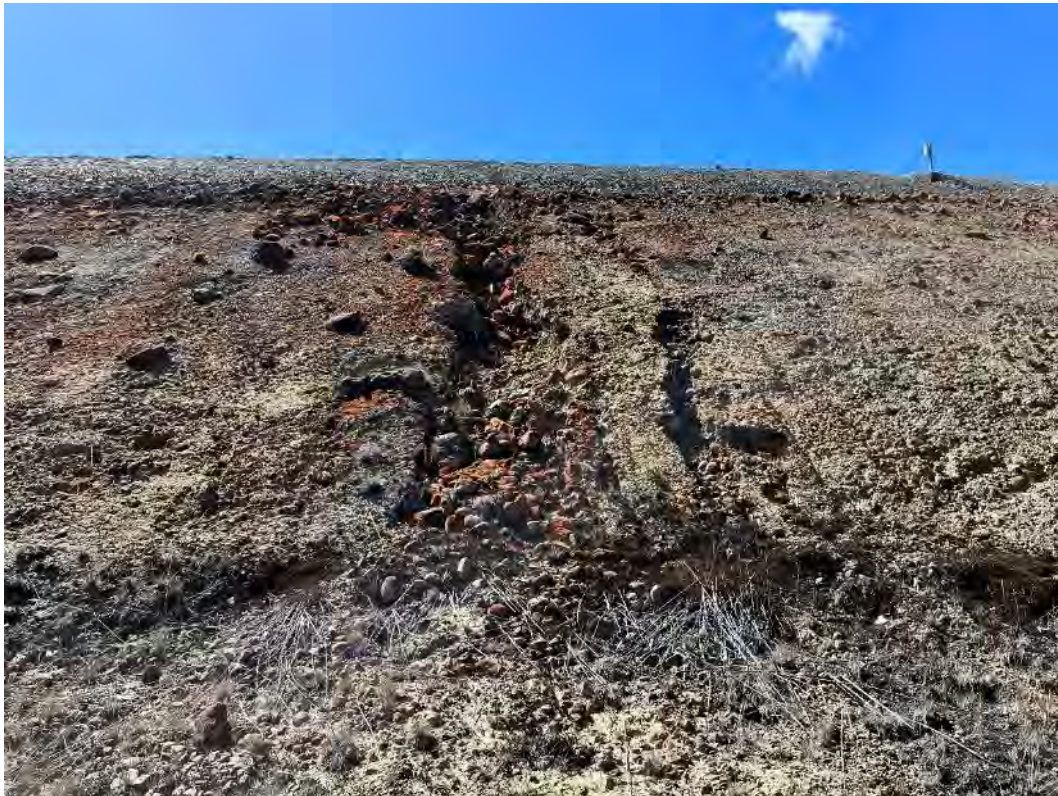
Photograph 13 – Erosion below Levee bench (typical).
