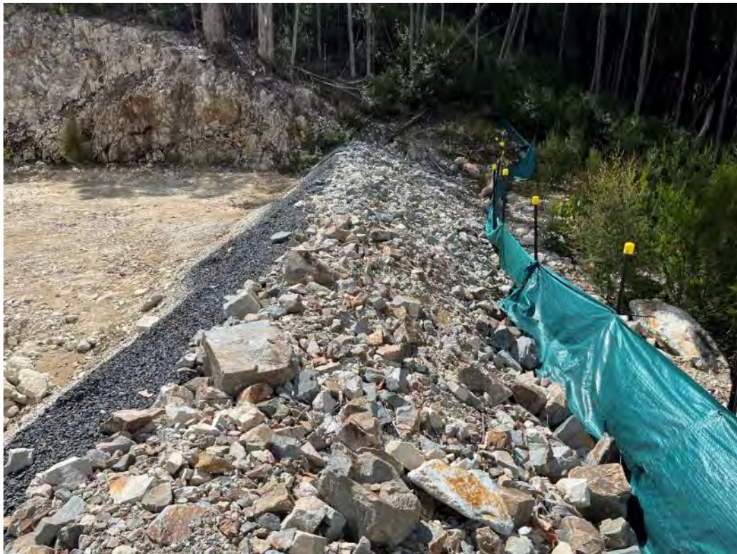
Photograph 31 – northern end of diversion channel. Note fill material placed for construction traffic will need to be removed once Stage 2 works are complete.
