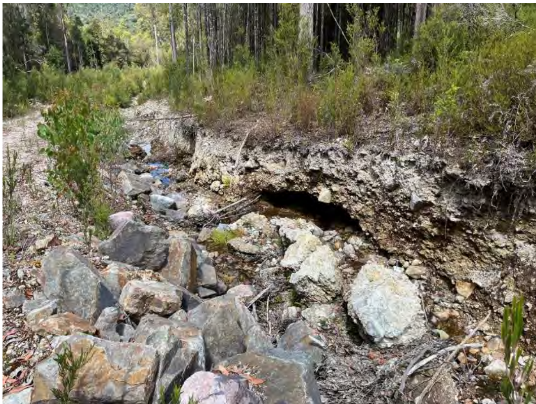
Photograph 2 – CWDD eroded upstream side slopes through glacial clays/silts. Does not interfere with water flow and does not affect access road profile. Has continued to slightly increase in extent compared to 2021 inspection.
