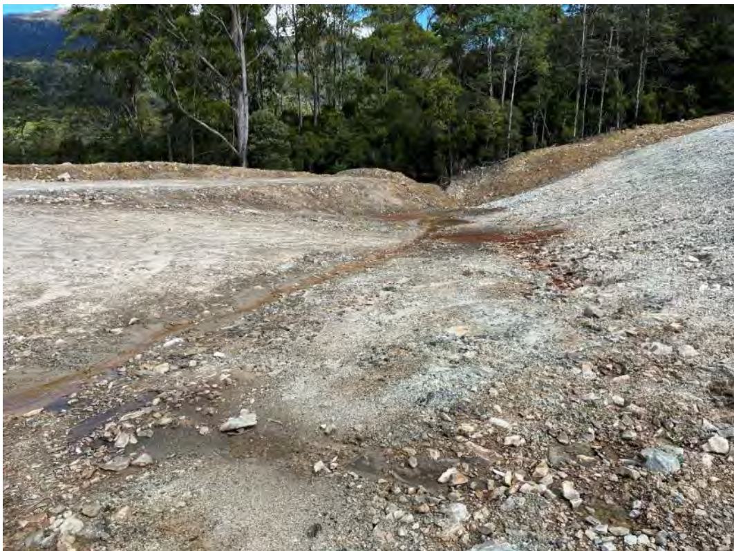
Photograph 12 – toe seepage from toe of original 5 Dam / 2 Dam interface.
