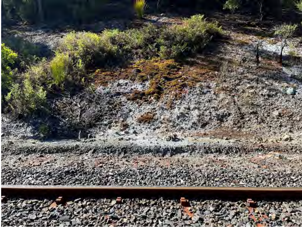
Photograph 7 -seepage and salt at toe of railway cutting
