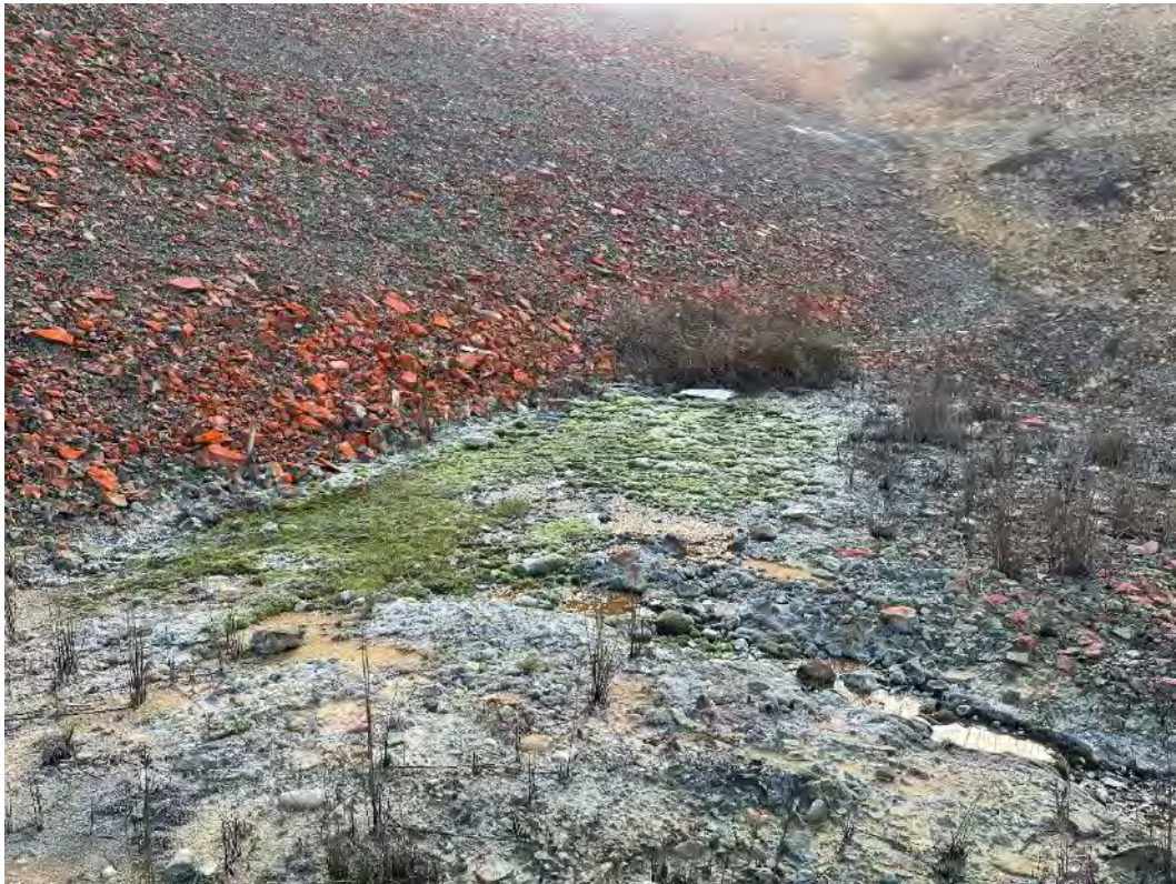
Photograph 33 – seepage from downstream toe of Southern embankment.
