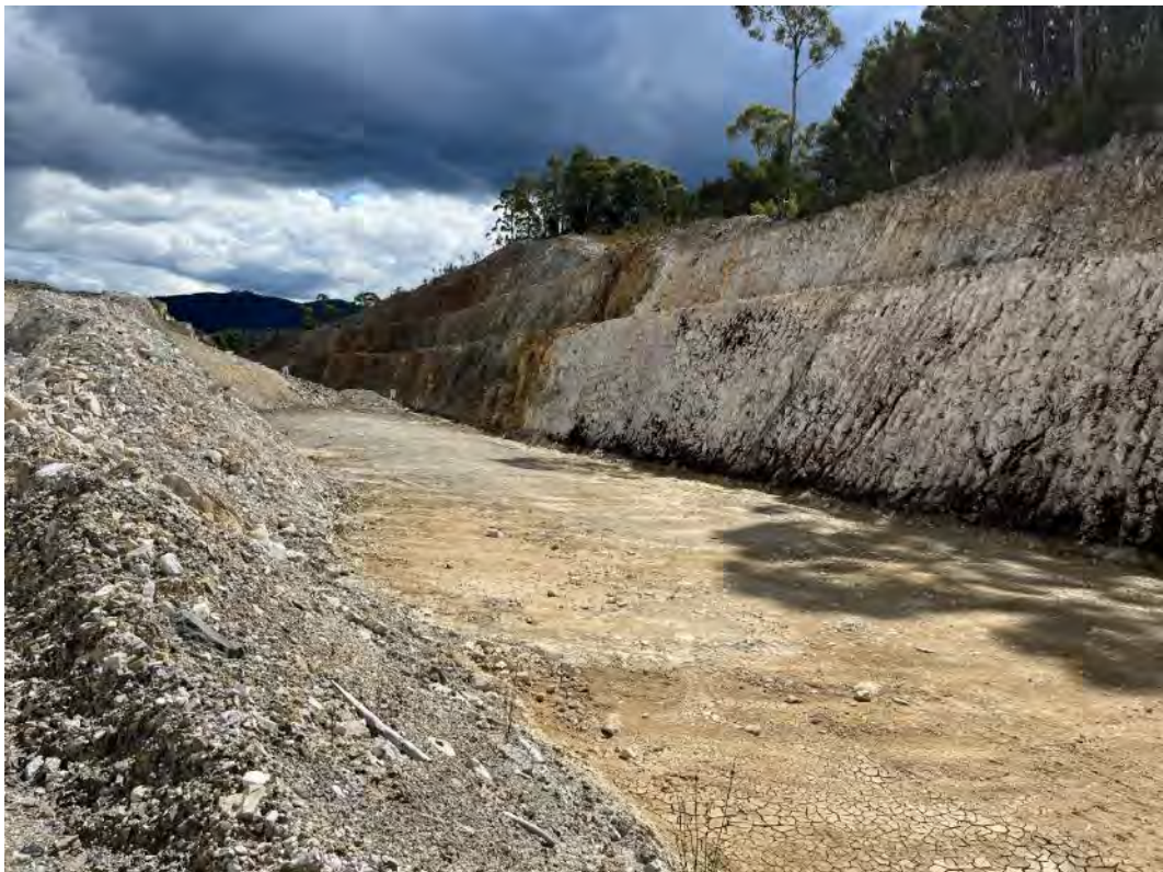
Photograph 30 – Diversion channel, looking south. Fill material placed to allow construction traffic to operate will need to be removed on completion of Stage 2 works.
