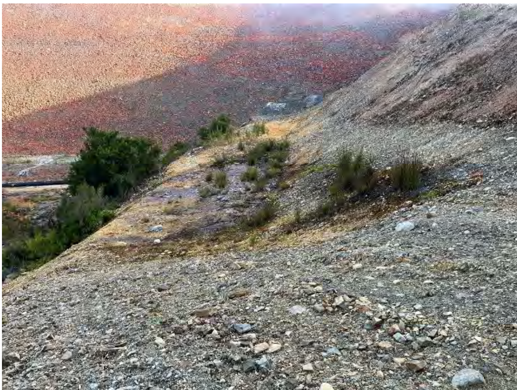
Photograph 34 – Seepage at southern access ramp, looking north.
