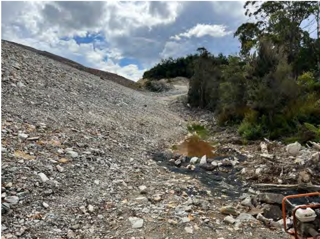
Photograph 9 – seepage at the western end of northern embankment.
