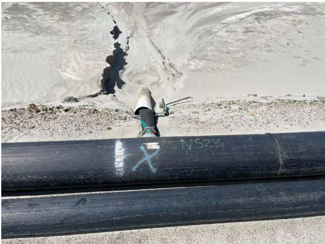
Photograph 24 – Typical slump on the upstream face due to rainfall and spigot conductor pipe spills
