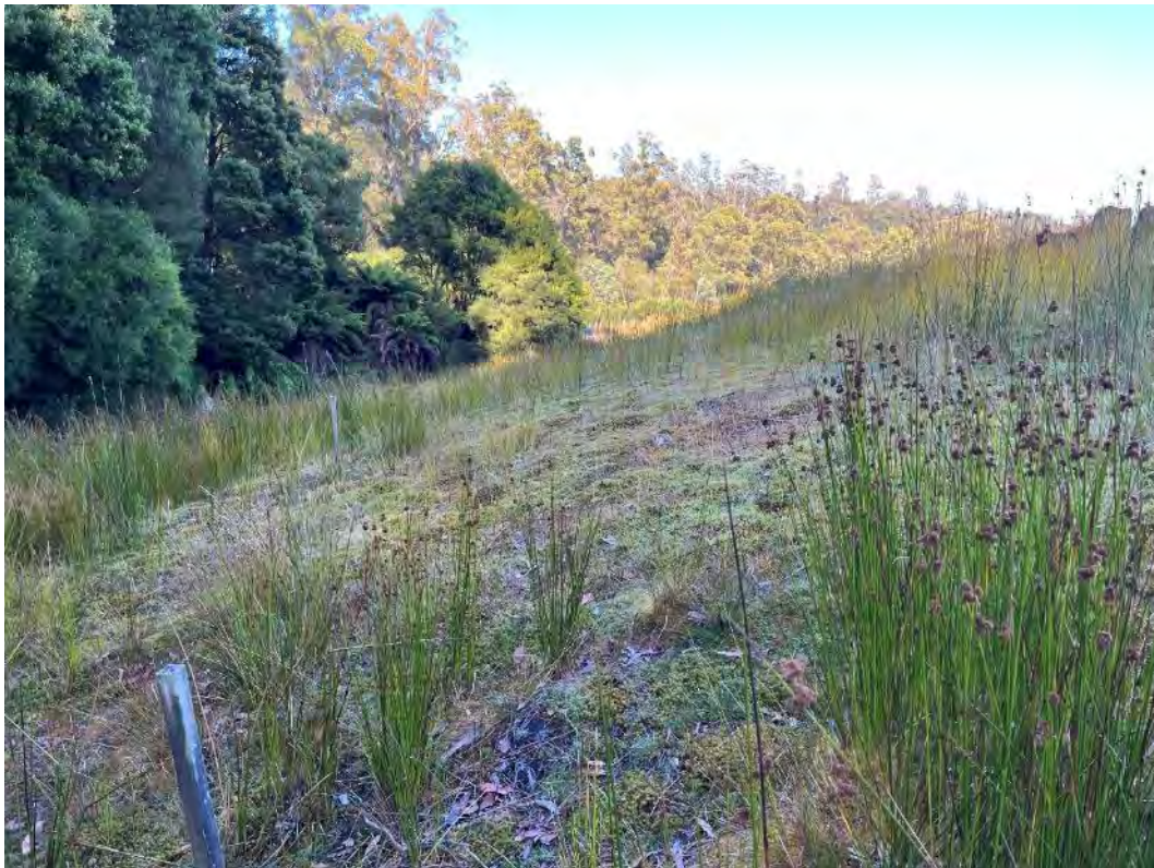
Photograph 43 – Polishing Pond – Old seepage point at the Northern end, below Decant 1– Moist at the time of inspection.
