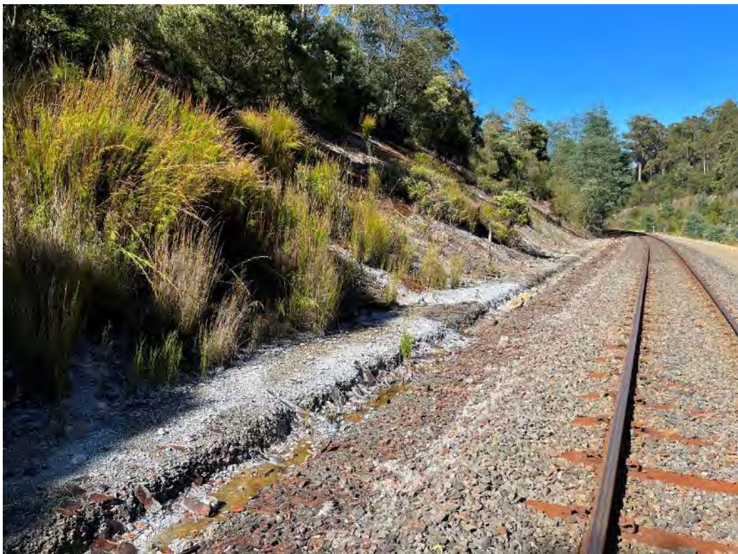
Photograph 6 – salt on railway cutting batter
