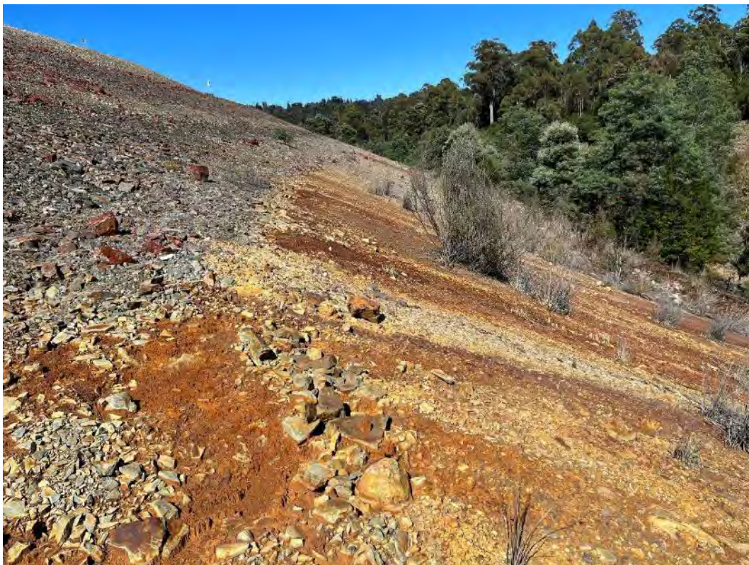
Photograph 14 – Iron staining on downstream slope of the Levee embankment, looking south. The iron staining is originating between the Stage 5/6 raises.
