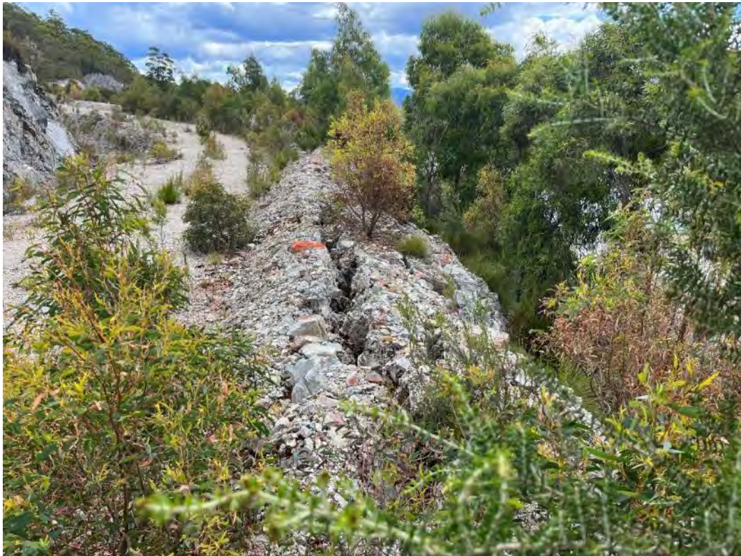
Photograph 3 – Condition of cracking in safety bund on downstream edge of CWDD.
