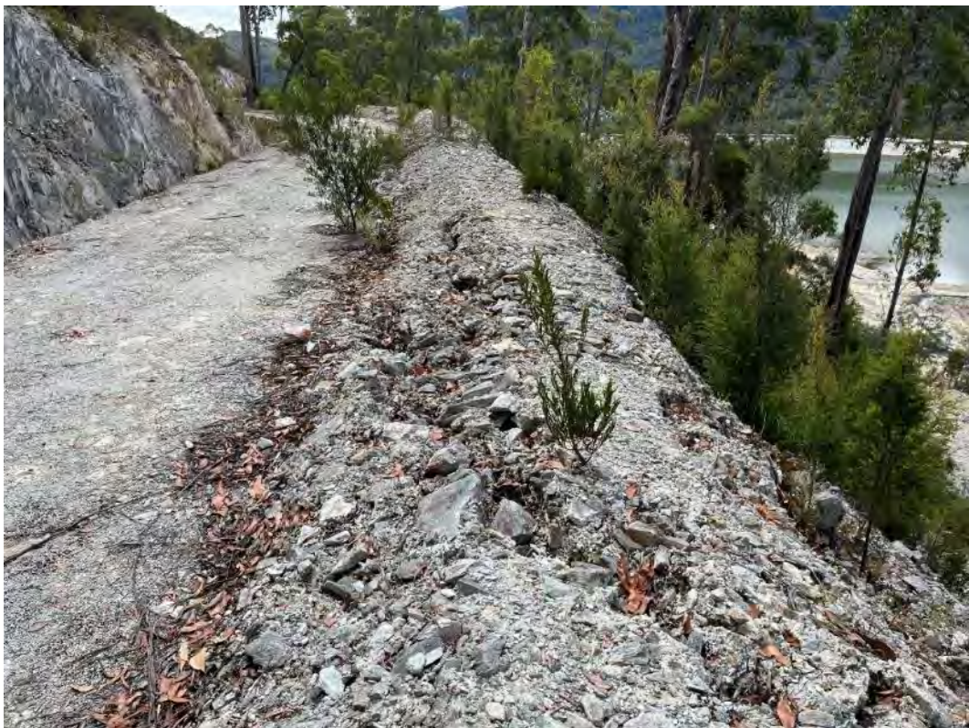
Photograph 4 – Condition of cracking in safety bund on downstream edge of CWDD.
