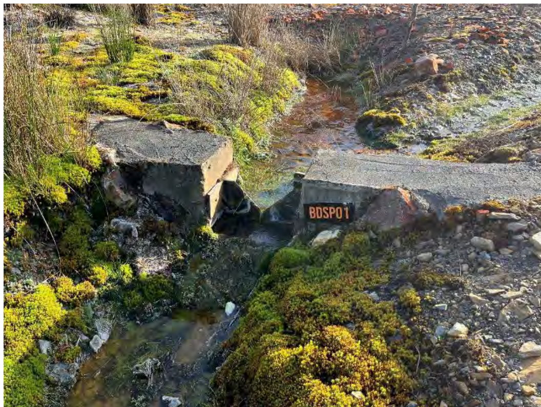
Photograph 35 – Moss and algae build around V-notch BDSP-01 requires clearing. Sediment build-up upstream of BDSP-01 should be removed.
