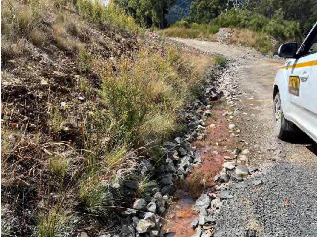
Photograph 5 – Concentrated clear seepage within old chimney drain outlet.
