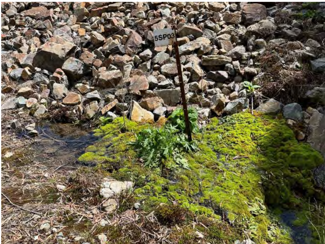
Photograph 10 – Toe seepage from original 5 Dam chimney drain outlet.
